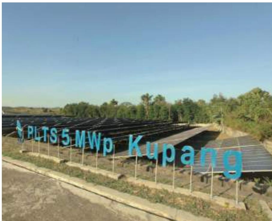
Image 3.2. Kupang Solar Power Plant in Oelpuah Village
